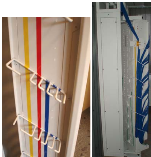
Patching frame pulled out and twisted
