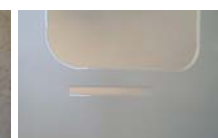
Notch in frame
