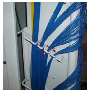
Patch cord in guides
