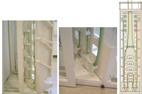
Cable at the rear of the frame
