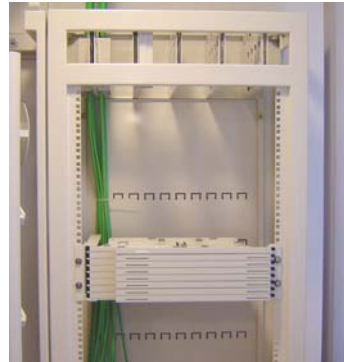
Location of splice module 1
